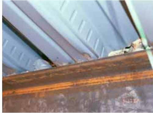
Figure 5.9. Local damage to Steel Deck Above the Top Flange
