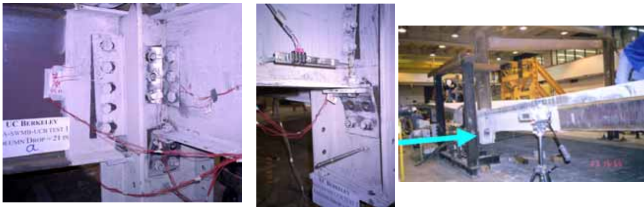
Figure 4.10. Loss of Two Bolts on the Seat Angle, Deformation of a Single Angle on the Web, and Free Rotation of the Beam in Slotted Holes
